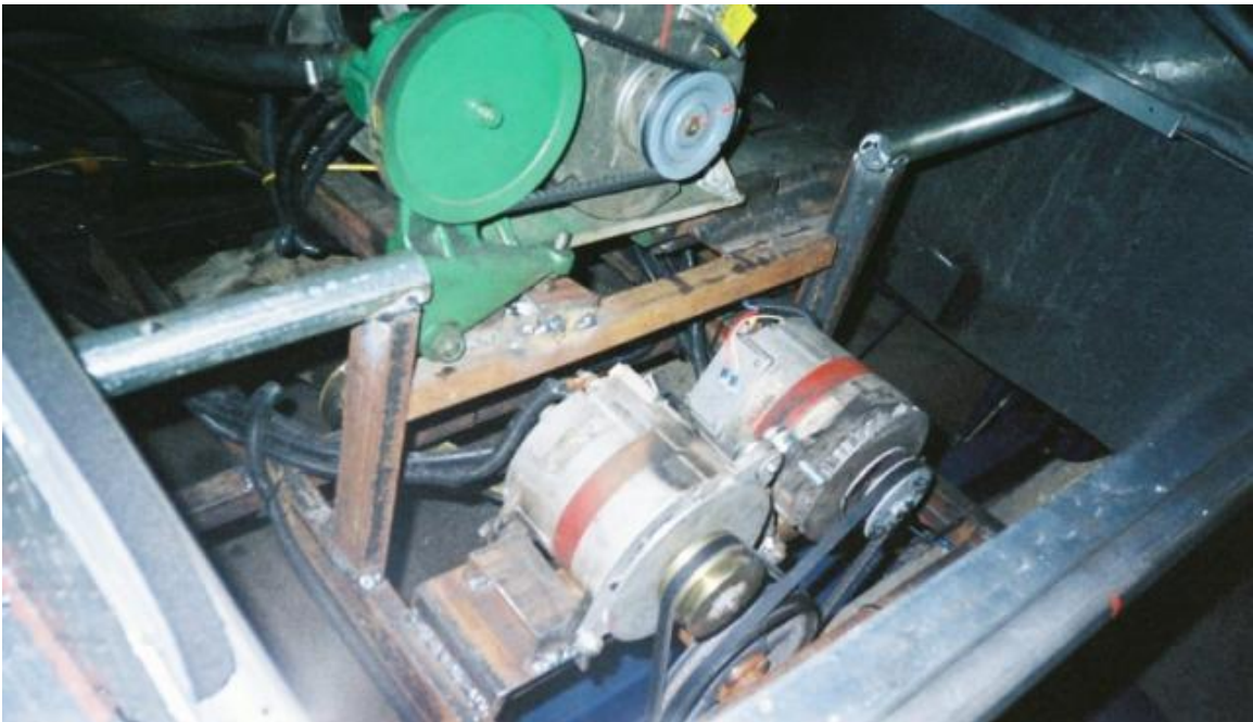
The alternators are for the auxiliary battery packs which feed the inverter.
