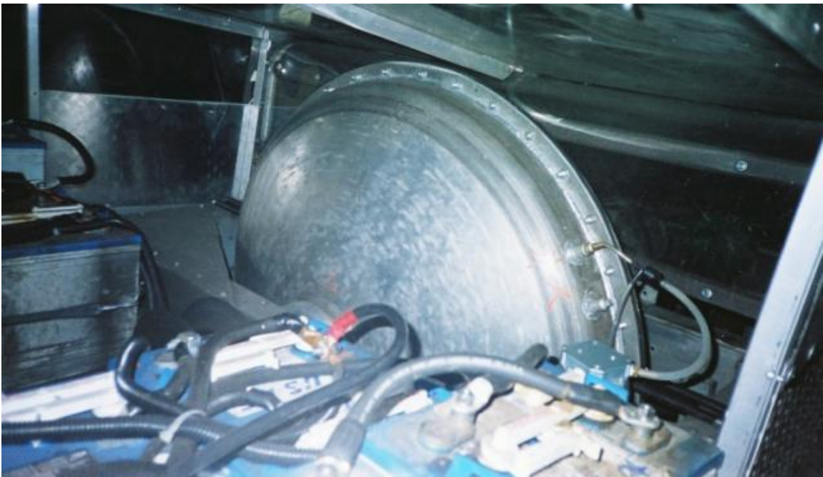
The opposite end of the flywheel chamber; Which is maintained under a vacuum. The batteries are for the auxiliaries.
